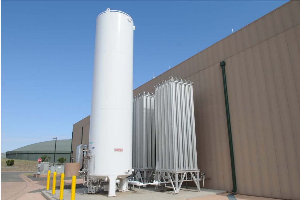
Figure 18. An Existing Liquid Oxygen Storage Tank and Vaporizers.
